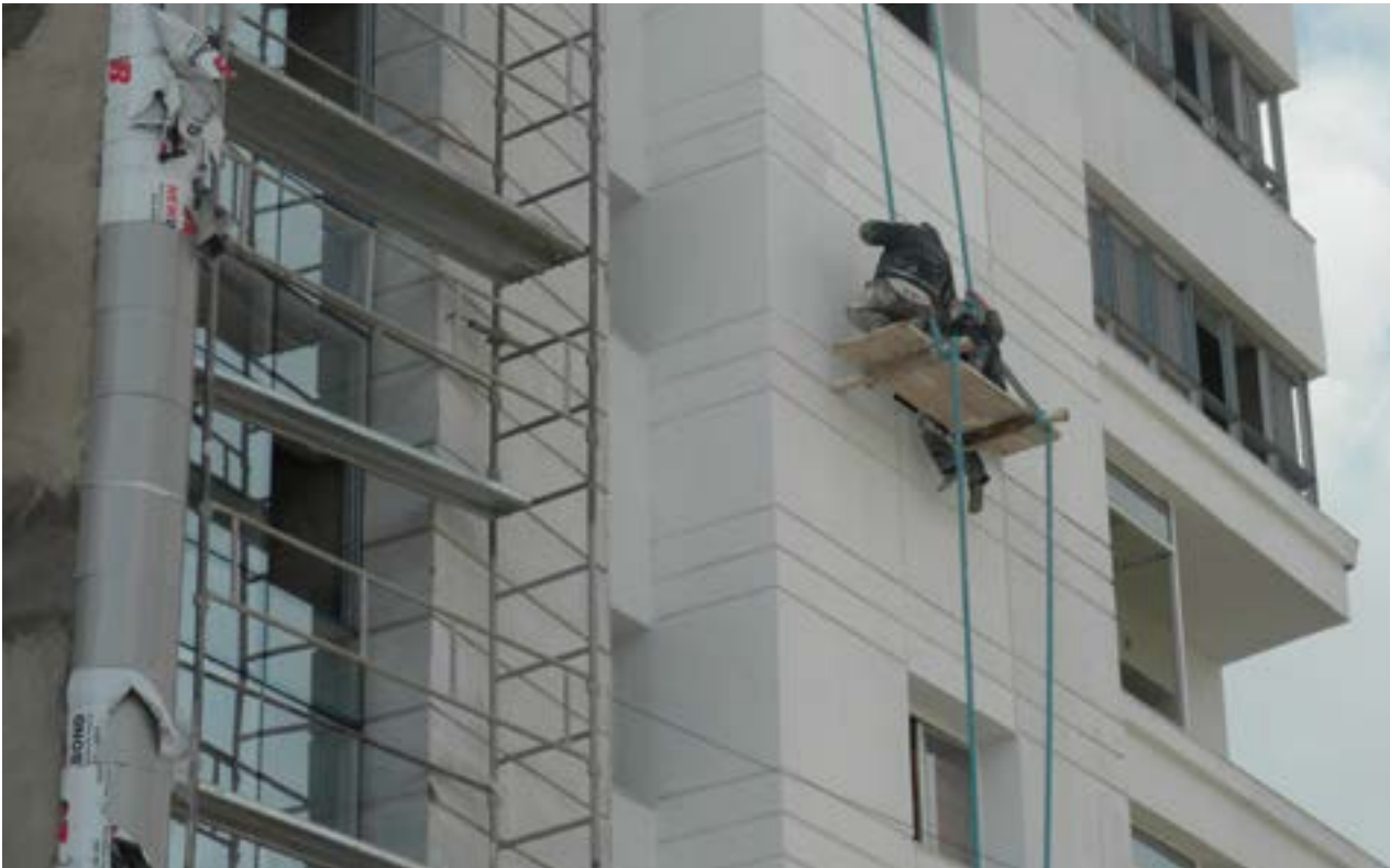
Construction workers work on a building in Tunisia with little safety protection. (Credit: Khaled Abelmoumen)
