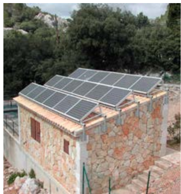
A sewage treatment plant that uses solar power on the island of Majorca in Spain. (Credit: Chixoy)
